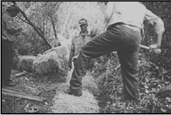
A work crew installing a straw bale fence as a sediment control measure to protect a riparian zone.
