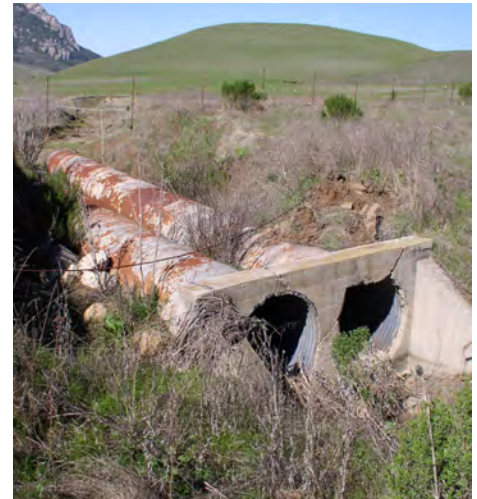
One of five old failed culverts that will be removed from Walters Creek to reduce erosion, restore a natural stream channel, and improve fish passage.
