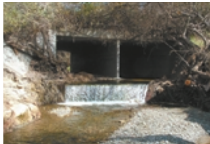
Barriers such as bridge crossings, culverts, dams and insufficient freshwater flows can block steelhead migration.
